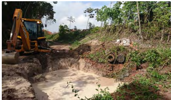
Photo 2: Inactive pipe outside the refinery. The area was excavated to allow the crack to be repaired.
