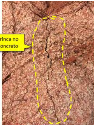
Photo 5: Detail of the cracked concrete.
